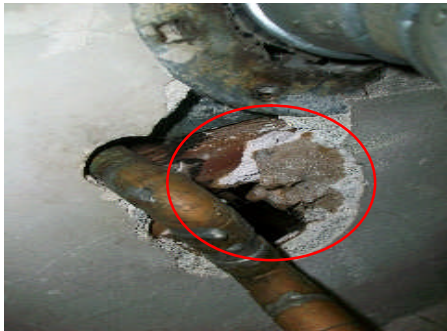
Water heater closet has holes around water Pipes need to be filled and sealed
