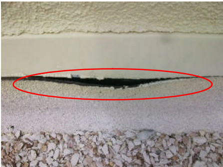
On roof next to balcony tar paper is separating from flashing
