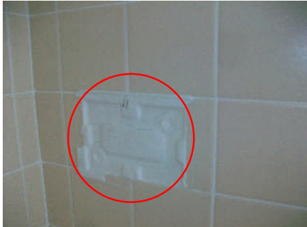
Upstairs shower soap shelf is missing
