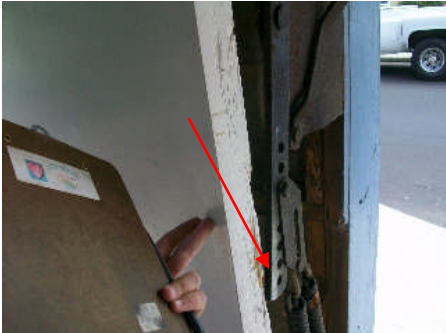
Garage over head door hard ware hits Garage service door
