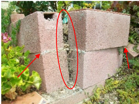
Garden retaining wall in front yard failing
