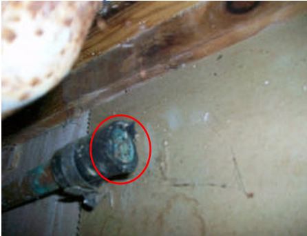
Pipe under kitchen sink needs to be capped
