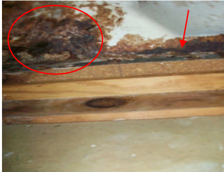
Under kitchen sink is rusting
