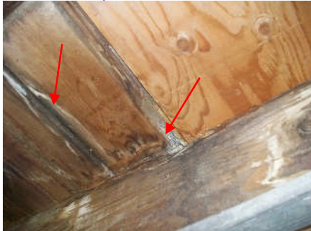
Garage roof has water stains and is leaking
