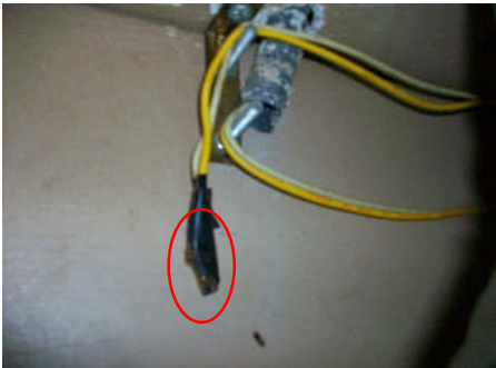
Kitchen hood vent cabinet has some exposed wires
