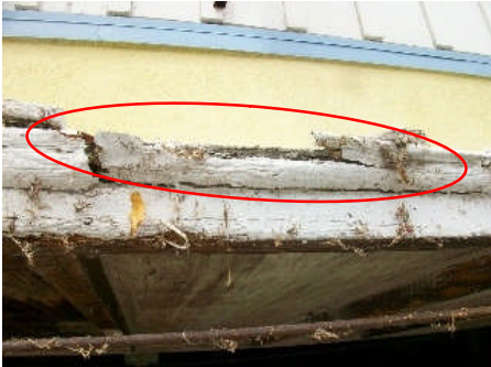
Garage weather stripping needs to be replaced
