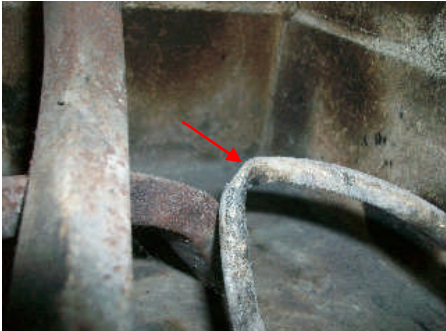
Dining room fire place gas line is kinked
