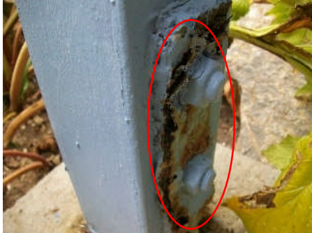
Deck support pier bracket is rusting out
