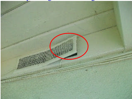
Attic vent needs to be sealed
