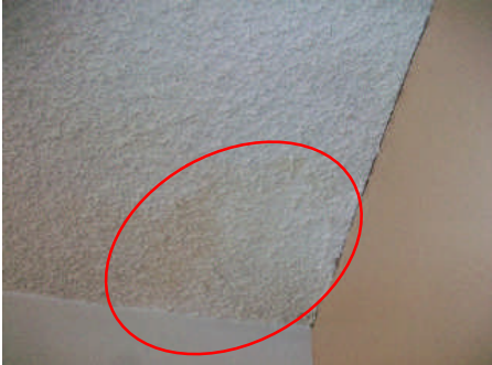
Moisture stain in living room ceiling
