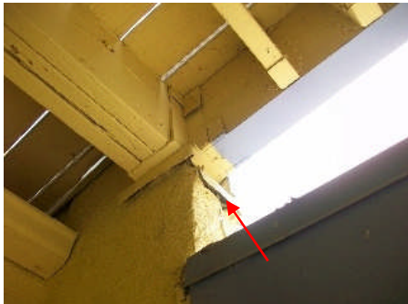
Under balcony hole next to flashing needs To be filled and sealed
