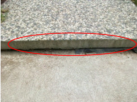
Concrete walk way has trip hazard
