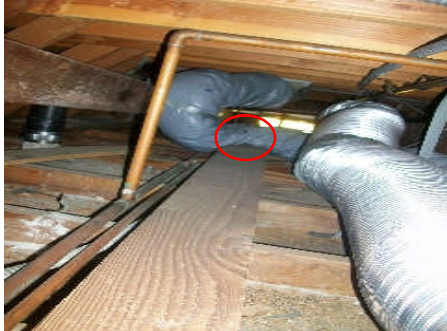
In attic HVAC ducting is collapsed
